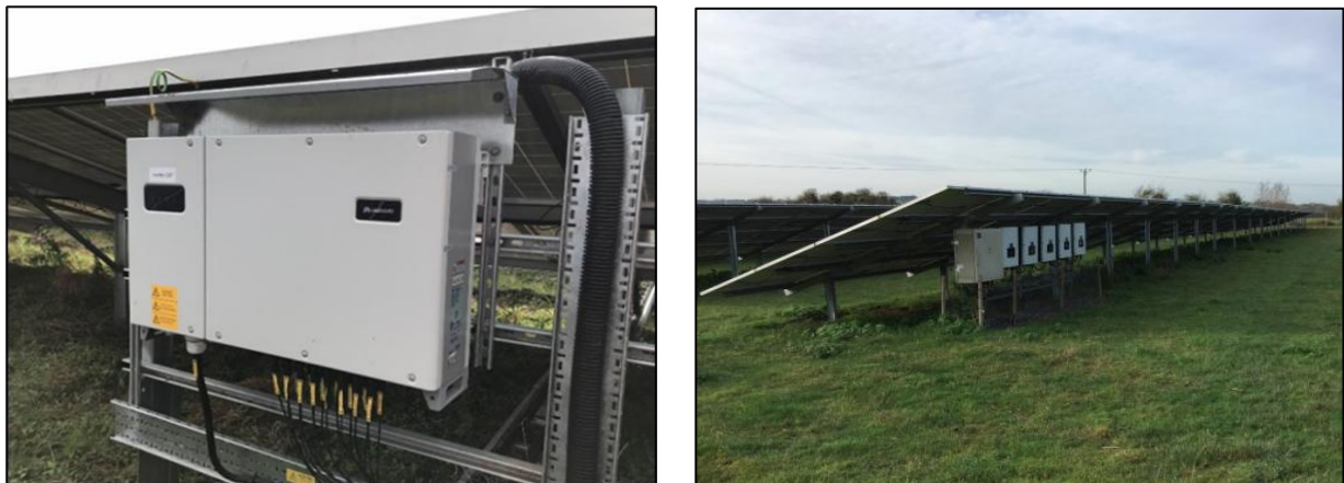
Plate 3.3 Typical String Inverter
